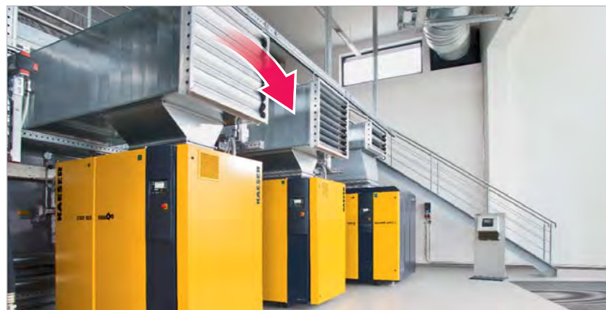
Fig. 3: Compressed air station with thermostatically-controlled air ducting
