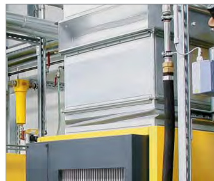
Fig. 2: Compressor ventilation connection with canvas duct joint
