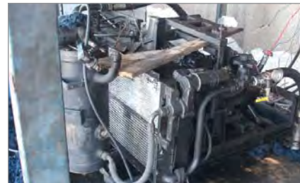
Fig. 1: Neglected compressed air station
